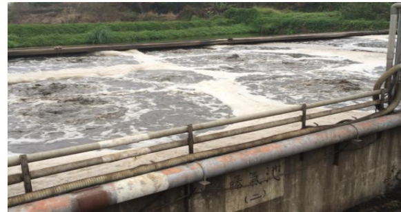
Activated sludge treatment
